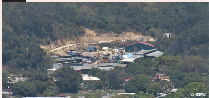
The cut slope and site formation work at Tai Kong Po which was suspected to have intruded into Lam Tsuen Country Park and is related to a STT granted by the LandsD
